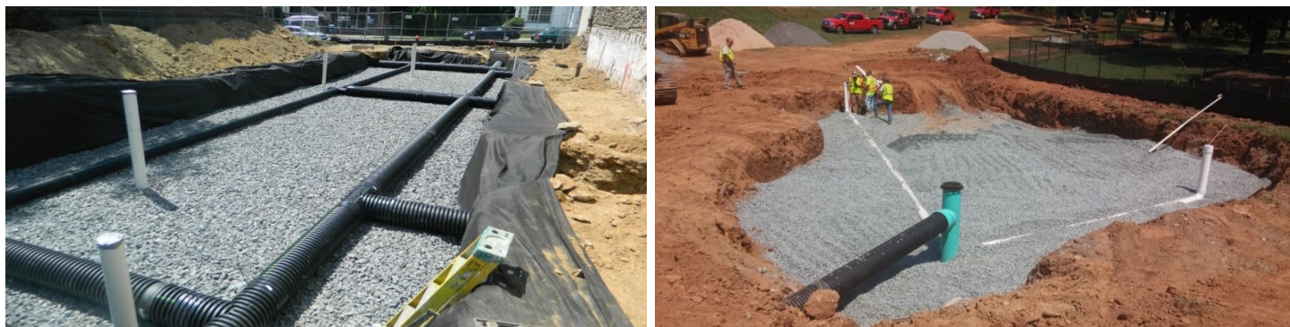
Left: SCM installation with HDPE underdrain pipe and capped PVC observation wells (Source: Philadelphia Water Department); Right: A bioretention area under construction in Salem, NC. Note the upturned elbow underdrain and capped cleanouts (Source: Hazen and Sawyer)
