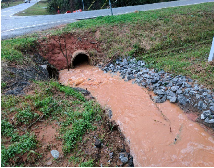
Figure 1.2.5.1 Excessive Sediment in Stormwater
