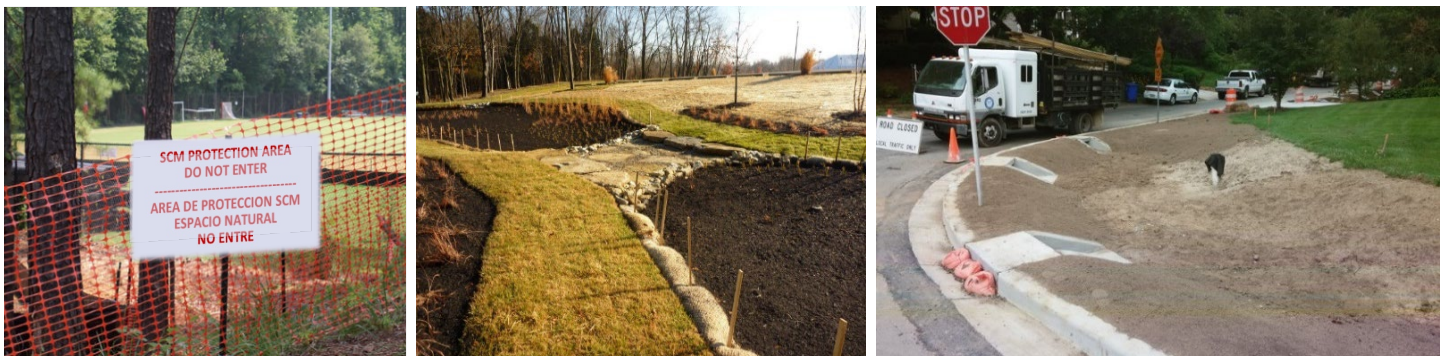
Left: A future bioretention area is protected during construction (adapted from a photo by North Carolina State University Extension); Middle: erosion prevention and sediment control measures surround this newly installed bioretention area until construction in the area surrounding it is fully completed. (University of Cincinnati’s Clermont College, the Water Environment Foundation); Right: Inlets are blocked to prevent inflows of stormwater during construction of a bioretention area. Note that all surrounding areas are fully stabilized. (Source: Montgomery County, MD Department of Environmental Protection)
