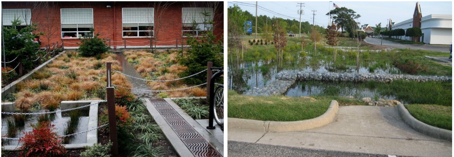
Left: A creative approach to forebay and inlet design is shown with the stilling-well type of forebay shown in the foreground on the left (source: Chachula Design); Right: A large forebay created by rip-rap gabion baskets, shown in the foreground of the picture, pretreats stormwater before it discharges to the main treatment area of the engineered wetland (Source: Center for Watershed Protection).
