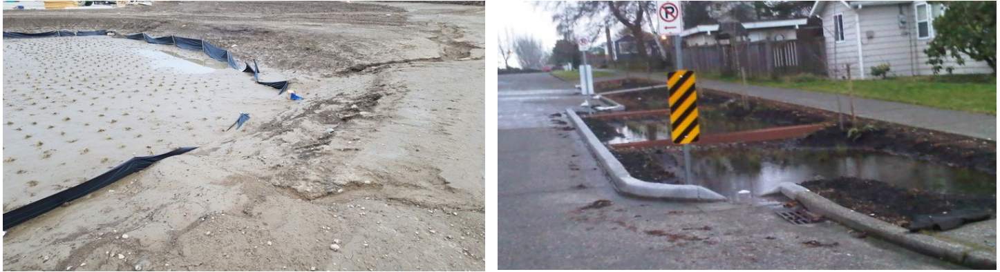
Figure 5.1.9.2 Results of Poor Land Disturbance Practices During Bioretention Area Construction
